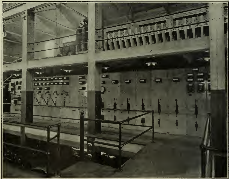
FIG. 13. GENERAL VIEW OF THE SWITCHBOARD
